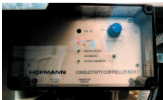
Conductivity meter: This meter measures conductivity of the water and controls a bleed-off valve to ensure the solids in the water do not exceed a pre-determined level
