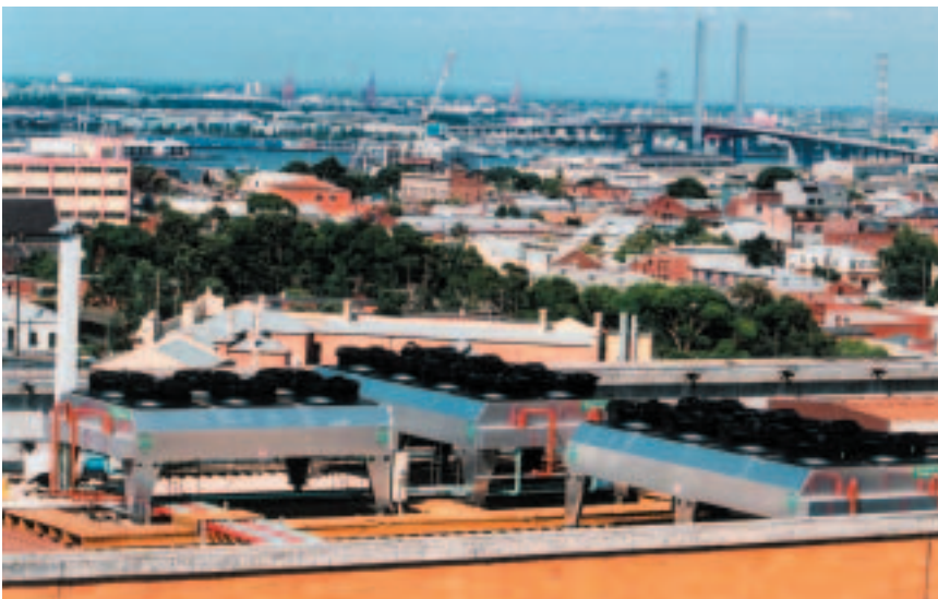
Air cooled system: Three air cooled systems forming part of an air conditioning system
