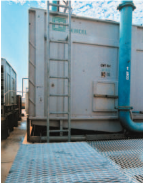
Tower ladder: Tower safety is important. Proper decking and ladders must be provided
